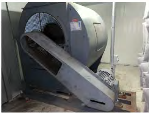
Image 33 – AHU 1.B Supply Air Fan/Plenum Before
