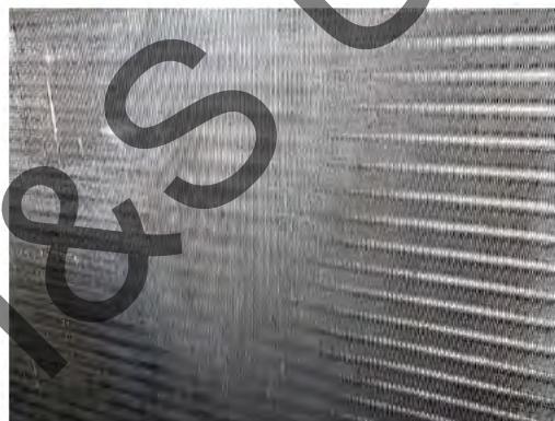
Image 24 – AHU 1.B Cooling Coils Air Off After
