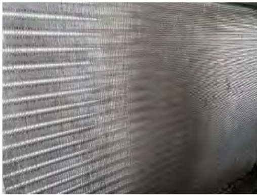
Image 21 – AHU 1.B Cooling Coils Air On Before
