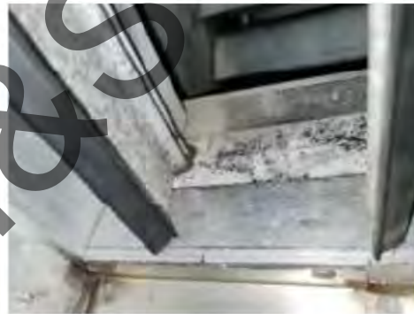
22. CTPI Plant Room (West Side) – Suspect mould on supply air dampers. Surface sample 111723B-T01-001 was collected here.
