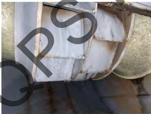
Image 31 – AHU 1.B Supply Air Barrel Fan Before
