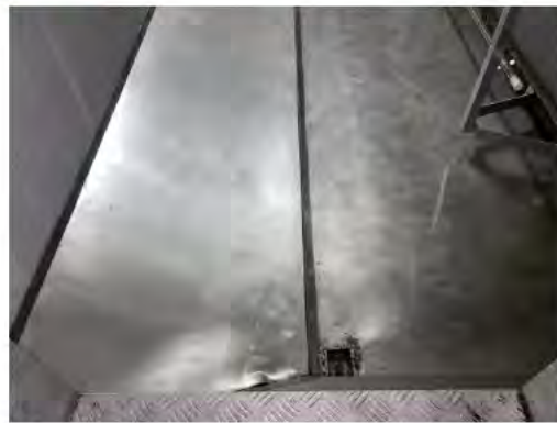
Image 26 – AHU 1.B Condensate Tray After
