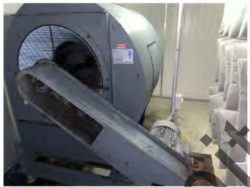
Image 34 – AHU 1.B Supply Air Fan/Plenum After
