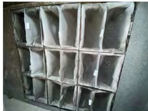
Image 20 – AHU 1.A Return Air Plenum Filters After
