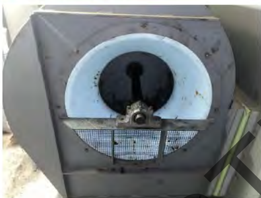
Image 35 – AHU 1.B Supply Air Fan/Plenum Before
