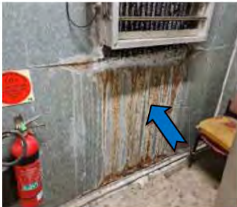
19. CTPI AHU Plant Room (East Side) – Visible corrosion was observed on the metal wall under the fresh air intake dampers.
