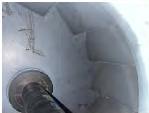
Image 8 – AHU 1.A Supply Air Fan Blades After
