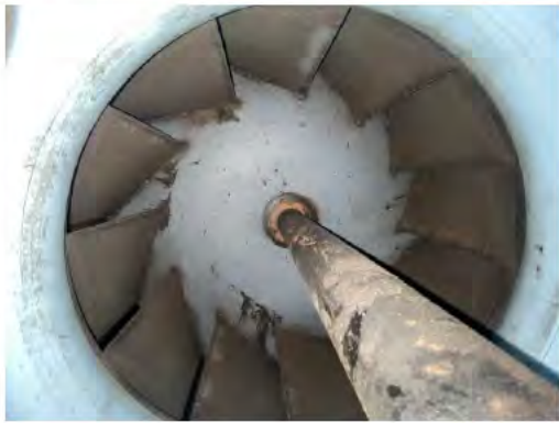
Image 27 – AHU 1.B Supply Air Fan Blades Before
