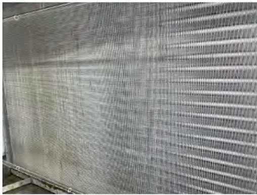
Image 3 – AHU 1.A Cooling Coils Air Off Before
