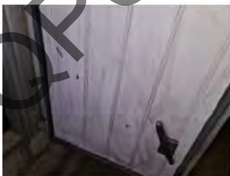
23. CTPI Plant Room (East Side) – Residual grime left from past cleaning efforts.
