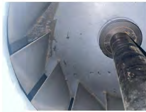
Image 9 – AHU 1.A Supply Air Fan Blades Before
