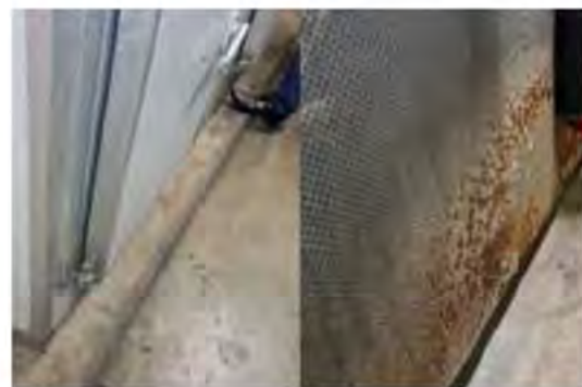
18. CTPI [redacted] Plant Room - The general area was observed to be affected by low levels of grime and dust, with suspicious mould spotting on pipework, joins, and connections. Further there was visible corrosion to metal walls, doors, latches, ductworks, and AHU housing.
