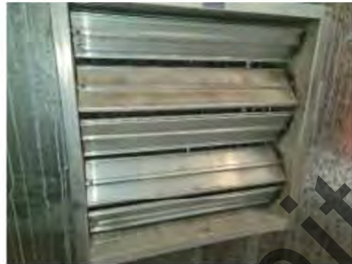
20. CTPI Plant Room (West Side) – The fresh air intake grill was noted to be mostly blocked by detritus (leaf matter, feathers, etc)
