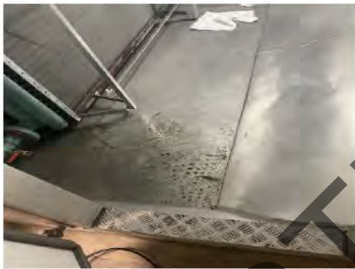
Image 5 – AHU 1.A Condensate Tray Before
