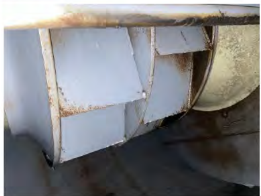
Image 32 – AHU 1.B Supply Air Barrel Fan After
