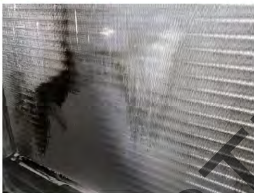
Image 23 – AHU 1.B Cooling Coils Air Off Before
