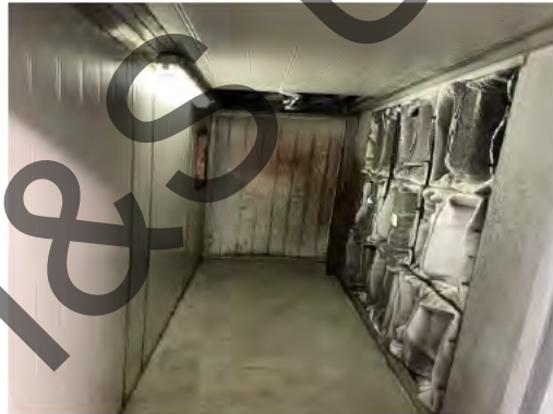
Image 18 – AHU 1.A Return Air Plenum After
