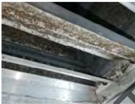
27. CTPI Plant Room – Grime and suspect mould on supply air dampers (AHU 1.B)
