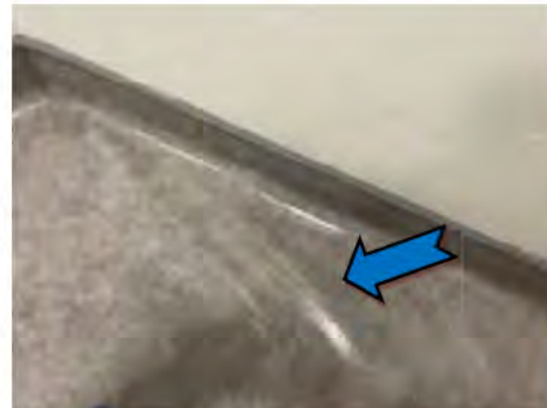
6. CTPI Locker Room – Vinyl floor located to the south-east side of the area, was observed to be warped/rippled.
