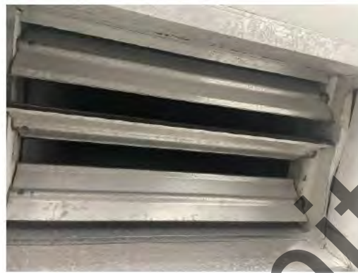
Image 16 – AHU 1.A Return Air Plenum After
