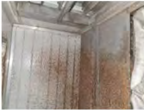
25. CTPI Plant Room – Representative corrosion in Mixing Chamber (AHU 1.A)
