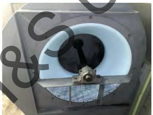
Image 36 – AHU 1.B Supply Air Fan/Plenum After
