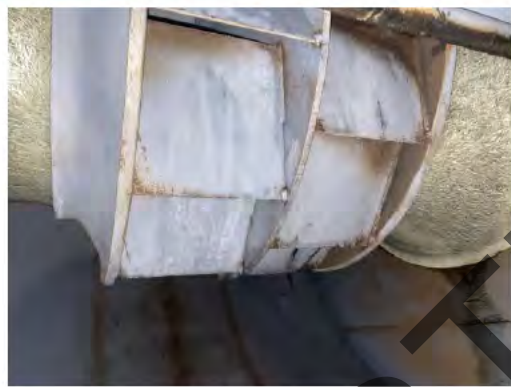
Image 11 – AHU 1.A Supply Air Barrel Fan Before
