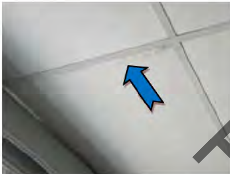
3. CTPI Education Training Office (ETO) – Ceiling tile adjacent window noted with dust staining.
