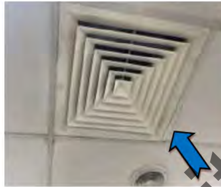
2. CTPI Education Training Office (ETO) – Air Supply register noted with dust loading.
