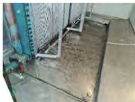
24. CTPI AC Plant Room (East Side) – Representative Grime and Corrosion in Supply Air Chamber & condensate tray
