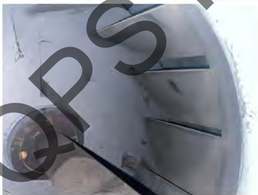
Image 7 – AHU 1.A Supply Air Fan Blades Before
