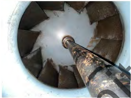
Image 28 – AHU 1.B Supply Air Fan Blades After
