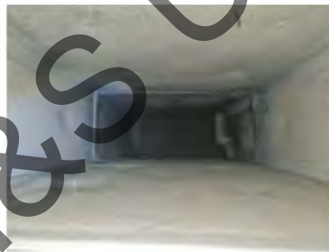
28. CTPI Plant Room – Supply Air Duct via inspection hatch downstream of Supply Air Chambers (AHU 1.A and AHU 1.B)
