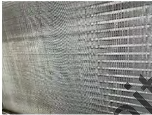
Image 4 – AHU 1.A Cooling Coils Air Off After
