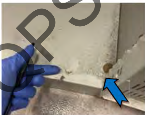
5. CTPI Locker Room – Dust loading was observed to shelving within and on top of personnel steel lockers.
