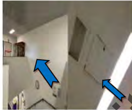
14. Foyer area CTPI [redacted], CTPI [redacted] CTPI [redacted] - Ceiling hatch observed to be swelling, with water staining observed to the plasterboard ceiling.
