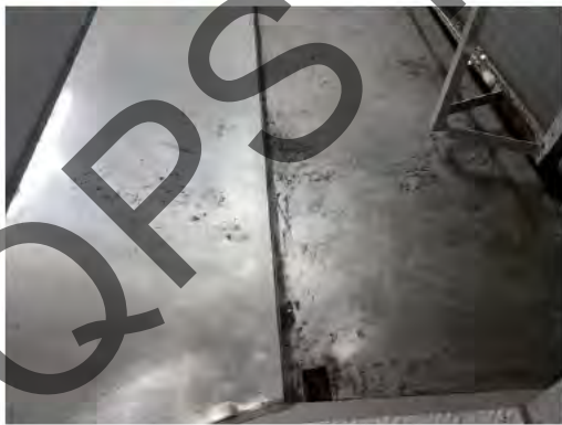
Image 25 – AHU 1.B Condensate Tray Before
