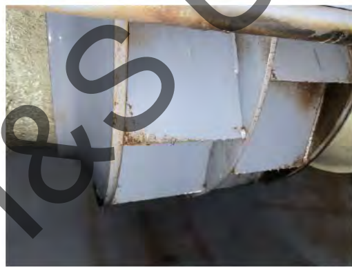
Image 12 – AHU 1.A Supply Air Barrel Fan After
