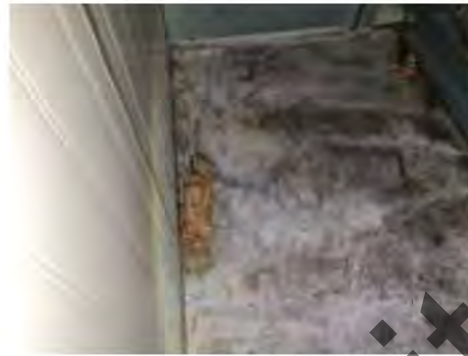
26. CTPI Plant Room – Rust and Grime in Fan Chamber (AHU 1.B)
