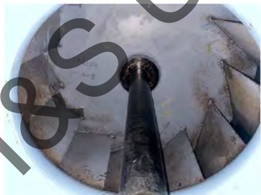
Image 30 – AHU 1.B Supply Air Fan Blades After
