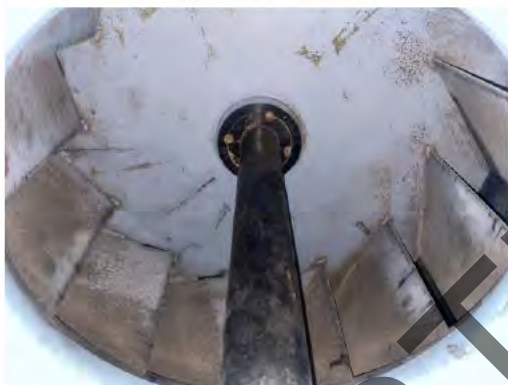
Image 29 – AHU 1.B Supply Air Fan Blades Before
