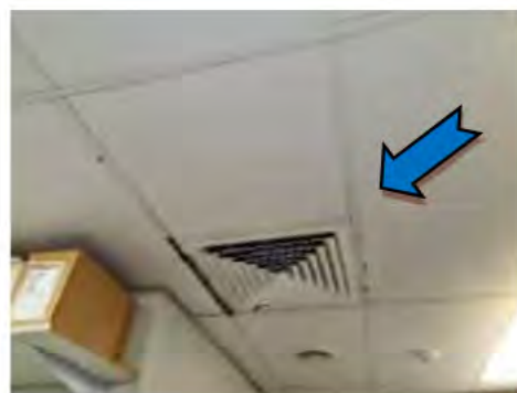
30. CTPI Scene of Crime (SOC) – Air Supply register observed to have dust loading with adjacent plaster ceiling tile noted to be peeling.
