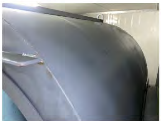
Image 38 – AHU 1.B Supply Air Plenum After
