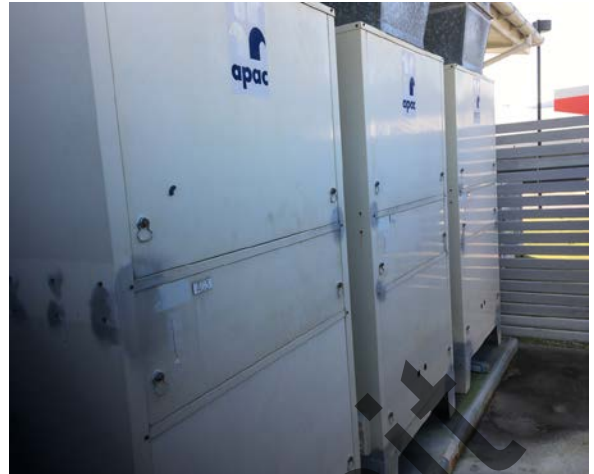
AC-1, AC-2 & AC-3 external condensers
