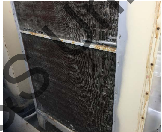
AC-1 condenser corrosion
