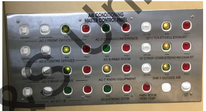
AC local master control panel
