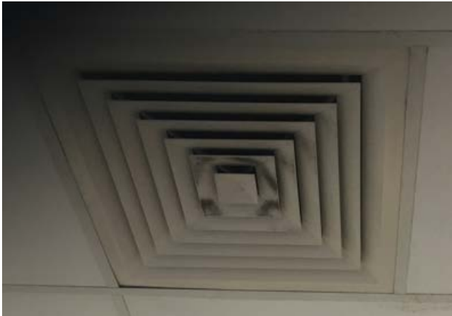
Typical ceiling diffuser with smudging
