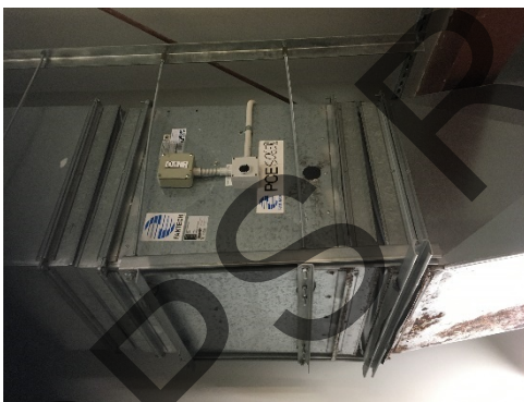
OAF-1 (duct corrosion on right)
