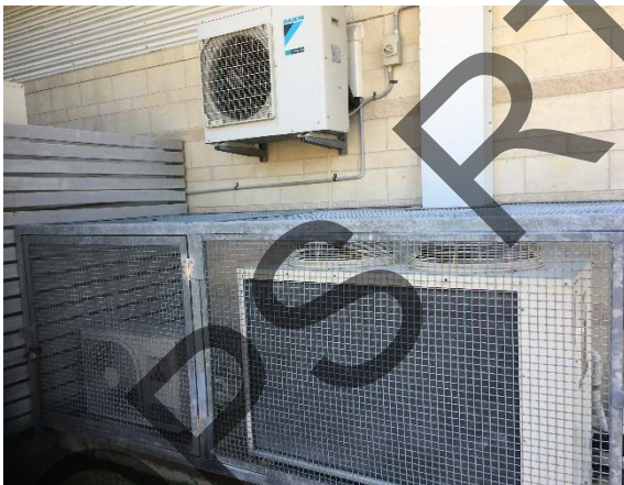
Other AC unit condensers
