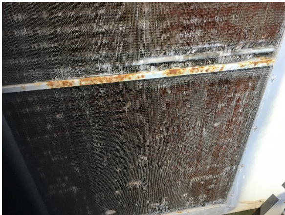
AC-2 condenser corrosion
